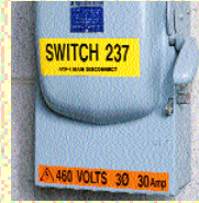
Panel & Switch I.D.
